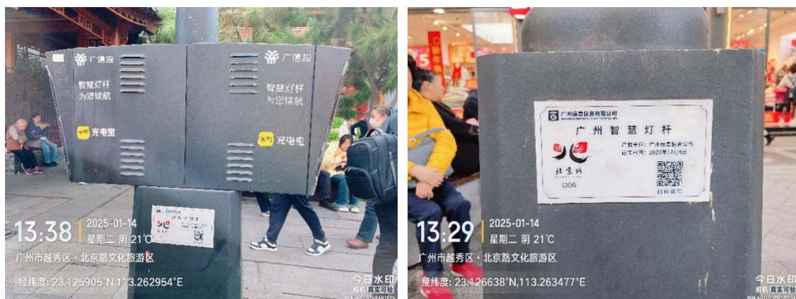
Figure 3-2: Existing smart lamp posts
