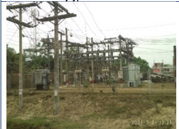
substation site at jagarnathpur, Thakurgaon PBS
