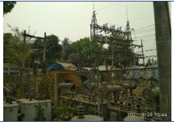
Substation Compound , Rangpur PBS-2
