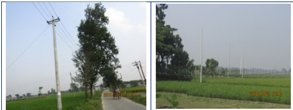
Figure III.3: BREB's existing distribution line
