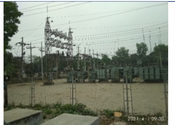
substation site at uttar Gobindopur, Dinajpur PBS
