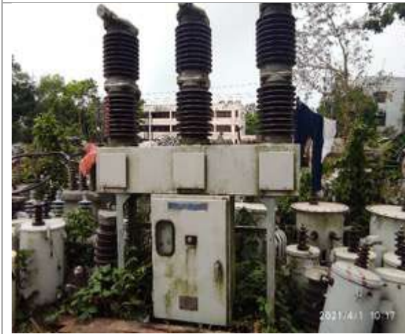
Transformers platform without spill control at Moulovibazar PBS
