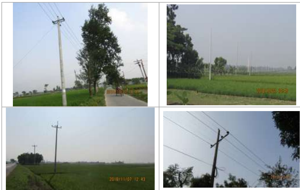
Figure III.4: BREB's existing distribution line
