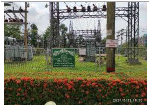
Laxmipur Sador 33/11 KV substation, Laxmipur PBS
