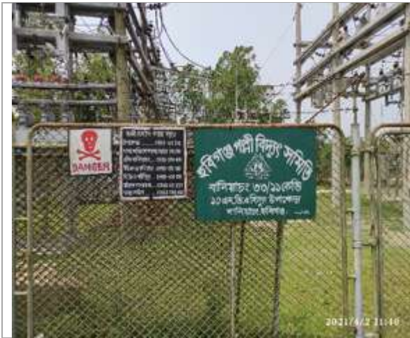
Baniachong 33/11 KV Substation, Hobiganj
