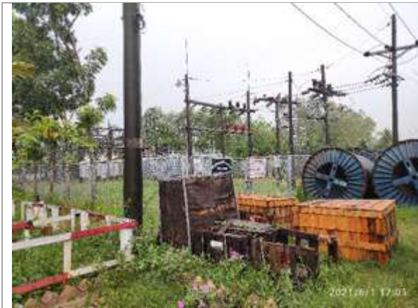
Sitakunda 33/11 KV substation, Chattogram PBS-3
