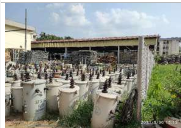
Old Transformers at Feni PBS
