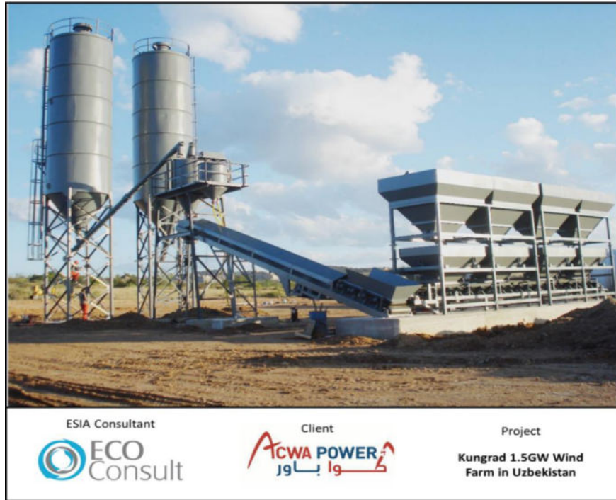
Figure 11: Typical Mobile Batching Plant
