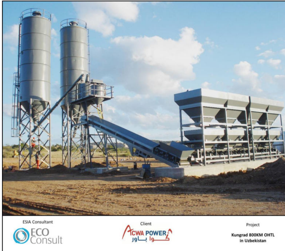
Figure 122: Typical Mobile Batching Plant
