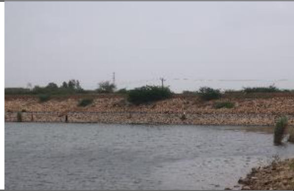
Water line on the embankment showing the highest level of the lake
