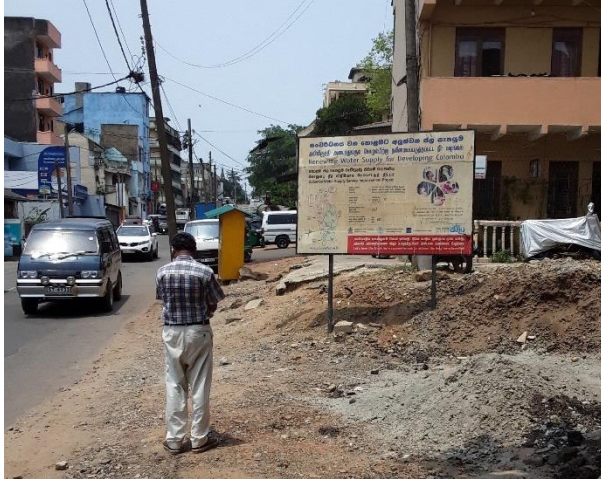
FIGURE 36 Water Supply pipe laying project and road widening project in progress along Aluth Mawatha (2021)
