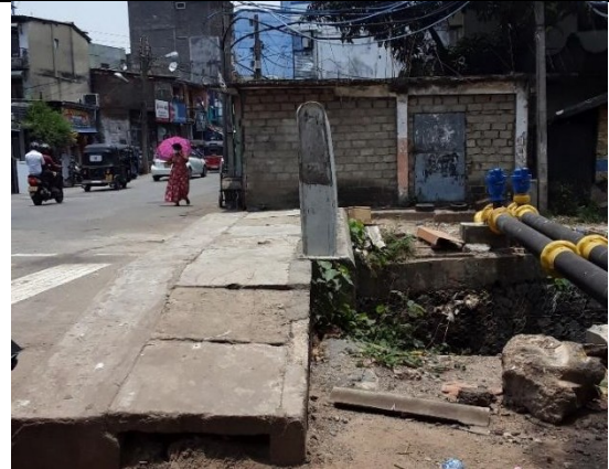
FIGURE 39 Bridge along the narrow section of Aluth Mawatha – Cables will cross this canal bridge
