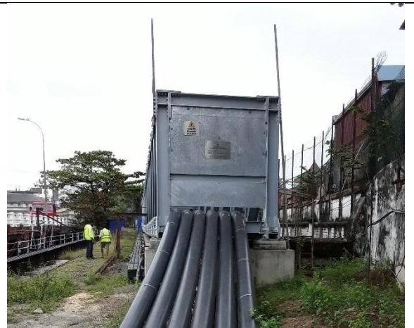
FIGURE 49 Cables already laid under Phase 1 along the road inside SLPP / New Hartal Bridge
