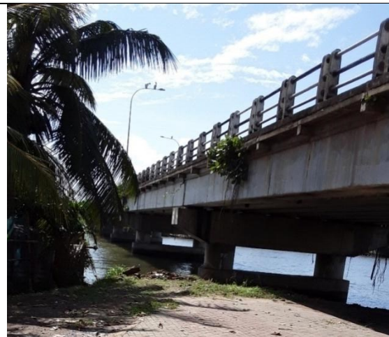
FIGURE 23 Mattakuliya bridge over Kelani River along the end of Old Negombo road (cable is already laid)
