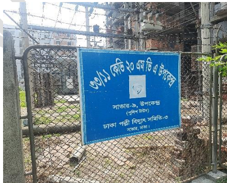
Figure 14-11 Grid Substation (Galaxy Apartment)
