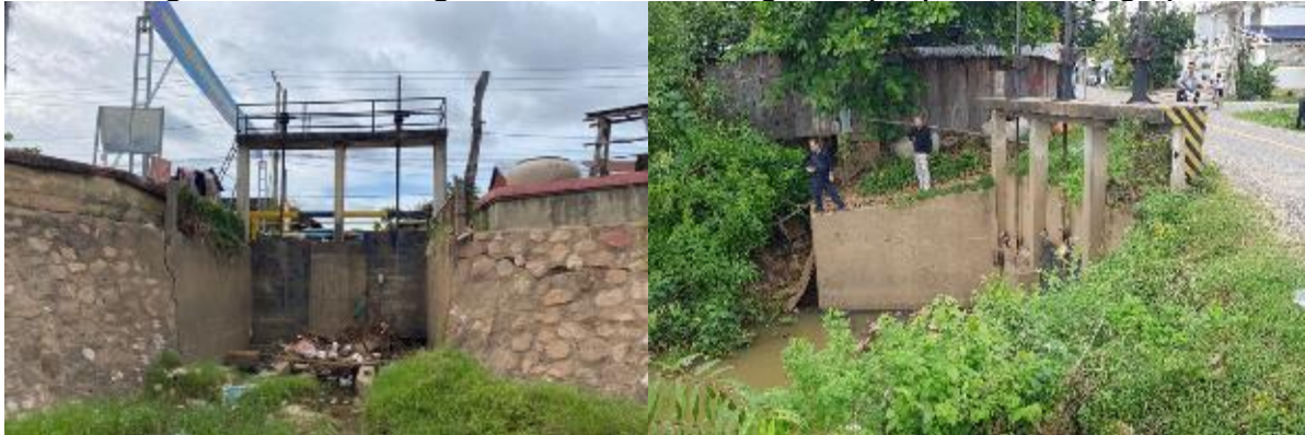
Figure I-4: Intake regulators for Kbal Hong MC1 (left) and MC2 (right)
