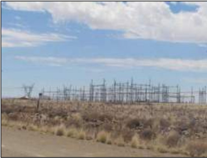
Figure 4: Aries substation 1 km south of the study area
