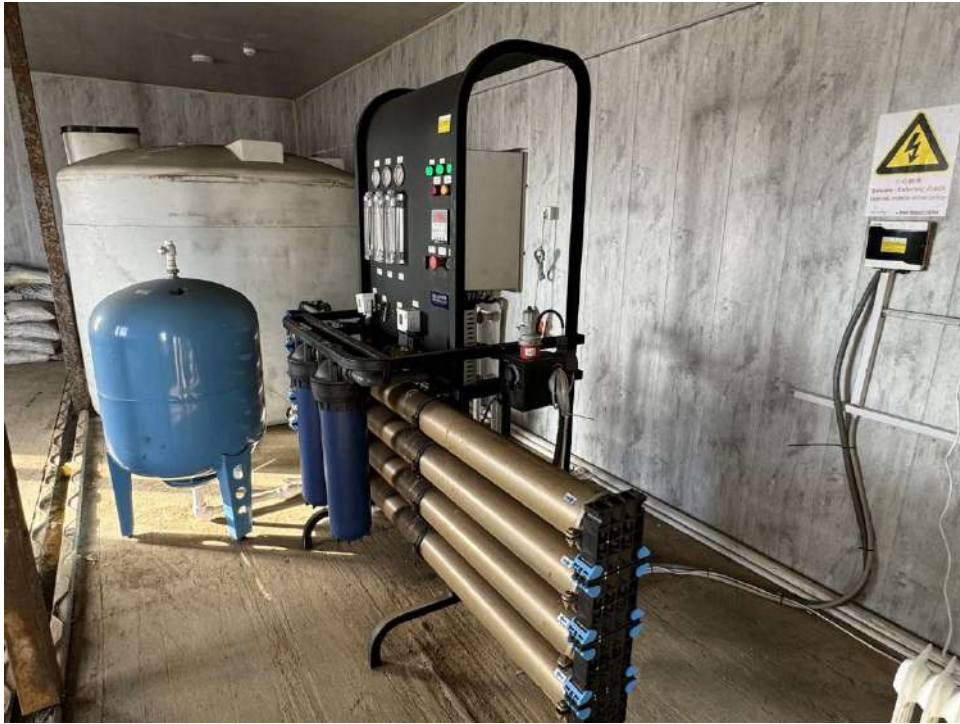
Figure 2-19 Existing Reverse Osmosis Unit in Place at the Nukus 1 WF Accommodation Area
