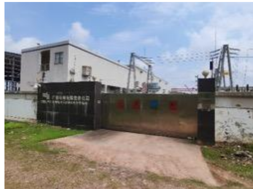
Linhu converting station
